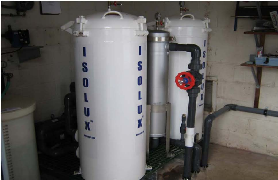
Figure 3. Isolux module installed in the well house.
