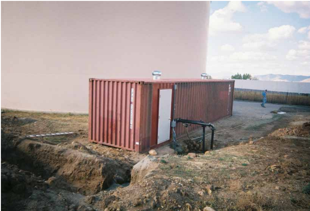
Figure 4-9. Isolux™ Treatment System Enclosure (Storage Tank in Background)
