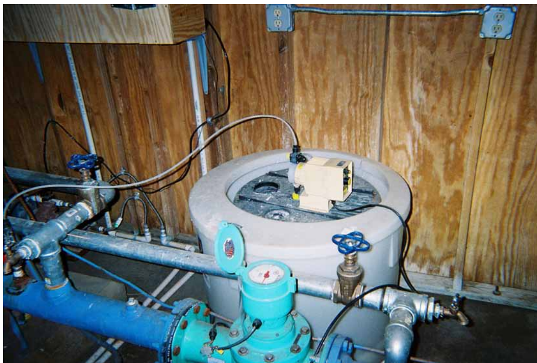
Figure 4-3. Pre-existing Chlorine Addition System
